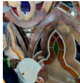
Old paint to the coloured glasses framework at the clerestory removed. Wood preservatives applied.
